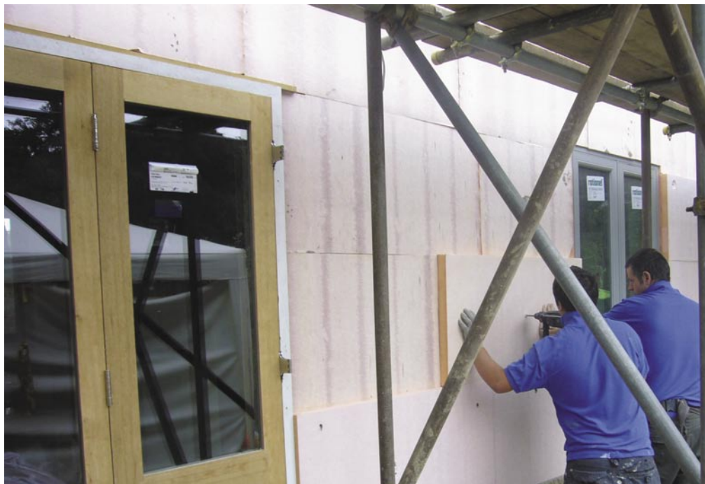
Above: the fixing of the external Permarock insulated render system over a 140mm thick dense concrete block wall meant a U-value of 0.15 could be achieved from a wall just over 300mm thick.
