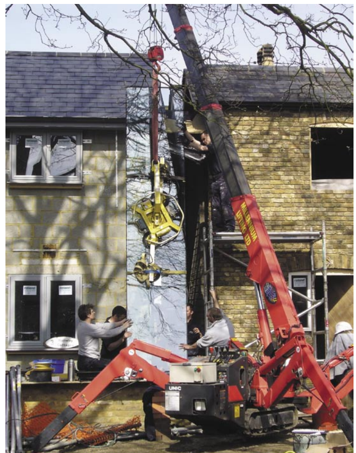
Above and far left: the main extension under construction and completed. Inset: the oak trusses on the roof which have proven to be a challenge with the airtightness expectations. Below: the placing of the novel glazed section that interconnects the old building to the new.
